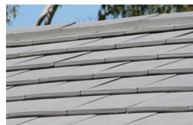
Top Ridge Shingle Roof
