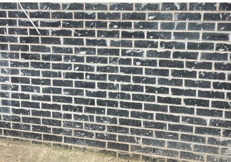
UNACCEPTABLE BRICKWORK AFTER LAYING
