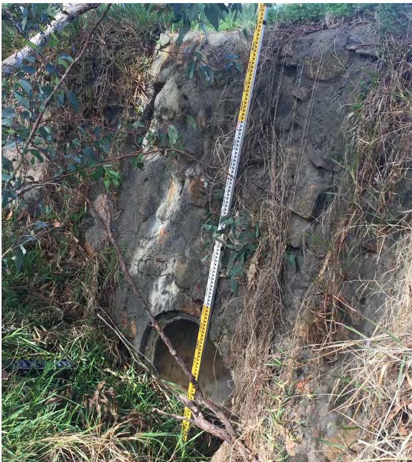
PLATE 8: 900 mm dia pipe under Muriel St. Invert of pipe is several metres below road level.
