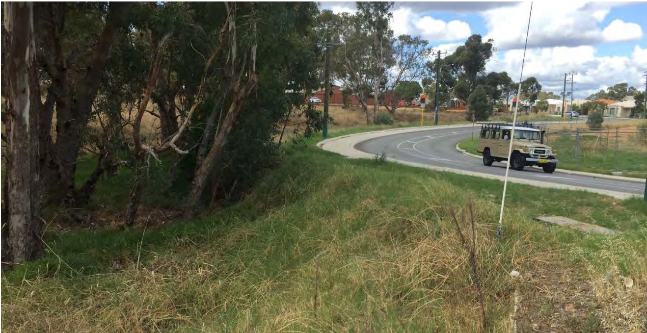
PLATE 7: Culvert under Muriel St at low point (approx. opposite vehicle location). Note Blackadder Creek Tributary is piped under development area immediately downstream of Muriel St.
