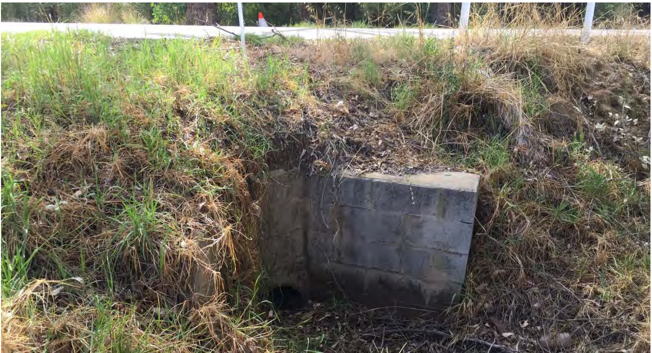
PLATE 2: Downstream end of 450mm dia Culvert under Eveline Rd. Partially blocked (50%).
