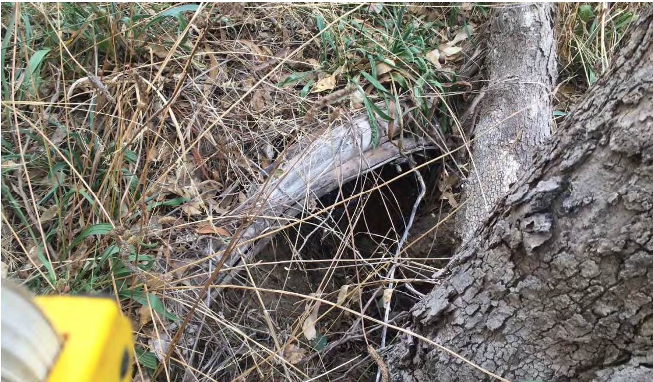
PLATE 4: 400mm dia steel culvert under driveway partially block by large tree.
